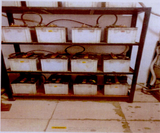
Server Room Battery section
